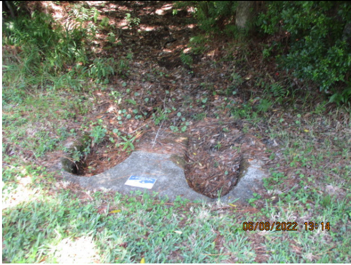
Image 13: MES/Pipes, silt build up, debris, needs clearing
