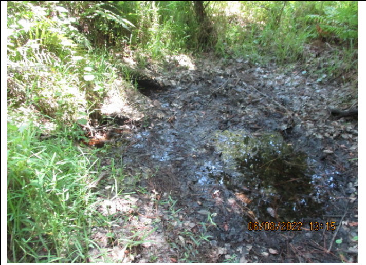
Image 14: MES/Pipes, silt build up, muck, needs Clearing, muck removal
