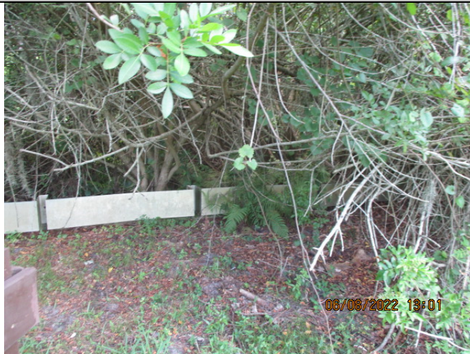
Image 9: Weir, Skimmer (rear yard) needs clearing
