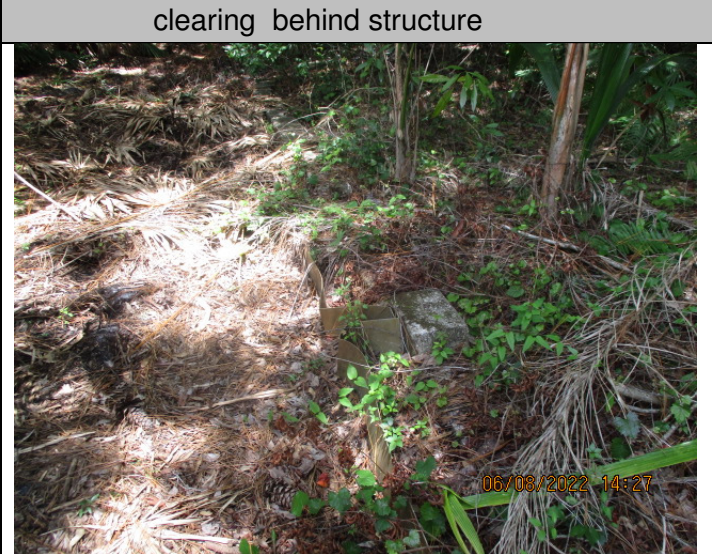
Image 12: Weir, Skimmer (rear yard) Barely Visible
