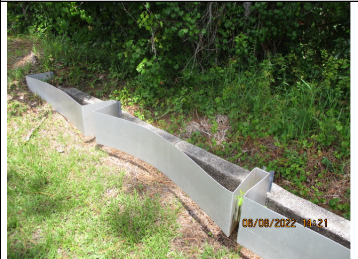
Image 10: Weir, Skimmer (rear yard) needs some clearing behind structure
