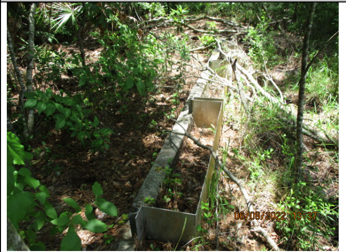
Image 4: Weir, skimmer need clearing, both sides
