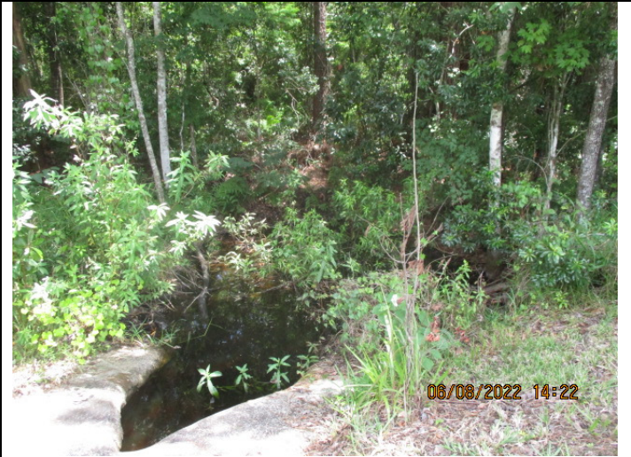
Image 16: Weir Structure, Skimmer west swale, needs clearing
