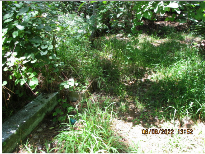
Image 5: Weir, Skimmer need clearing, both sides
