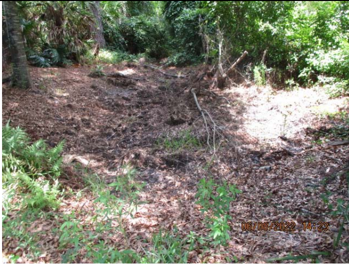
Image 15: Inlet basin/ Grate completely covered with silt, debris, needs clearing
