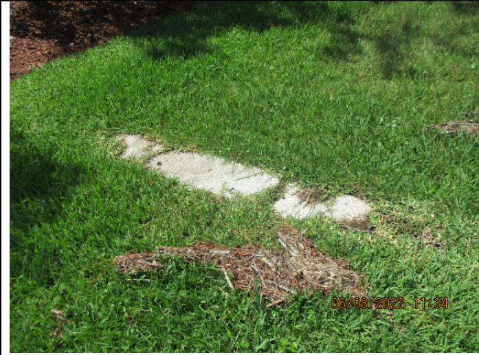
Image 6: Ditch check (weir) silt build up & Vegetation in roadside swale
