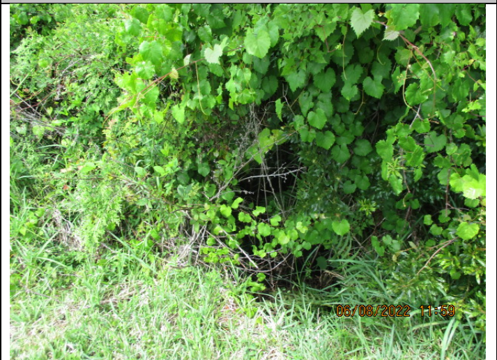
Image 12: Connecting Fes/Pipe on opposite side of road barely visible, needs clearing
