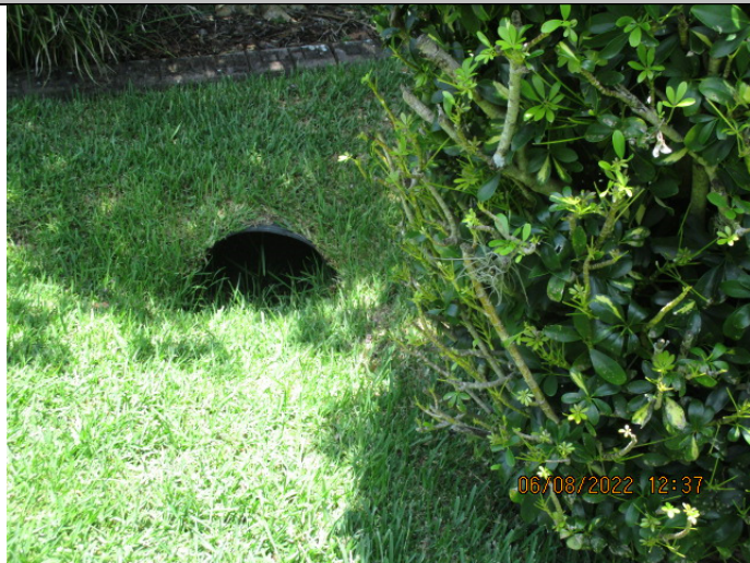
Image 17: Pipe in connector system under rod
