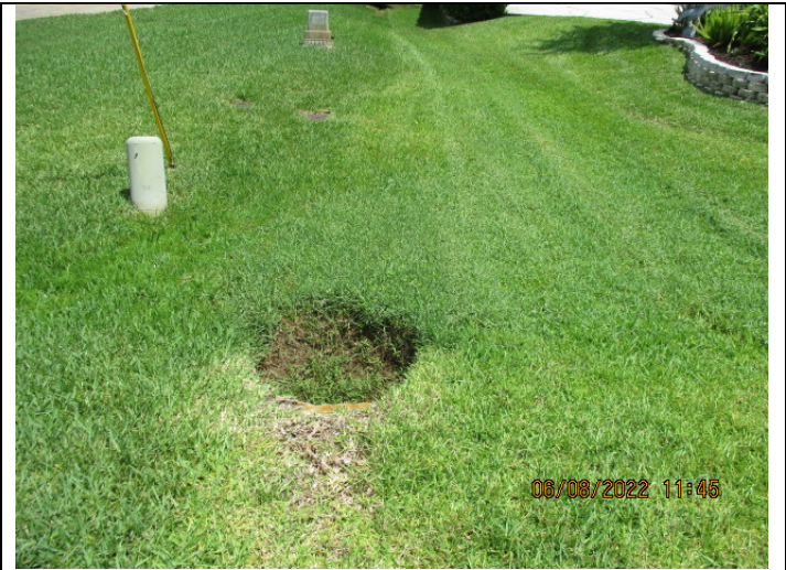
Image 8: FES/Pipe in swale that flows to wetland excessive silt & vegetation build up at pipe end
