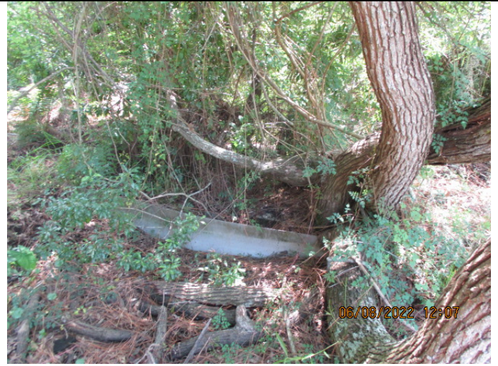
Image 14: Weir Structure, Skimmer east swale, needs clearing
