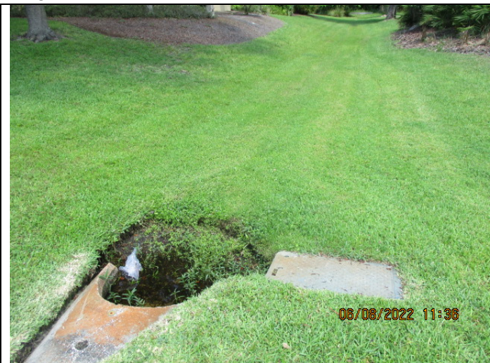
Image 2: FES/Pipe discharges to wetland via swale excessive silt & vegetation build up at pipe end.
