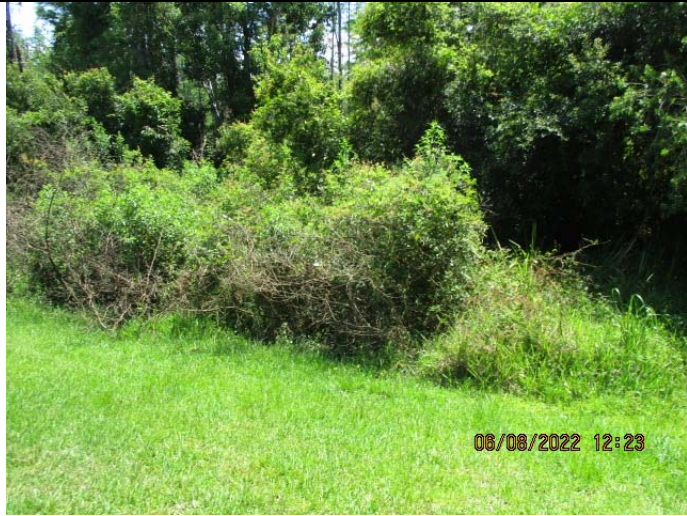
Image 15: Weir Structure, Skimmer east swale, completely overgrown, needs clearing
