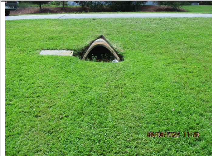
Image 3: Opposite view, swale filled in should be to bottom of pipe
