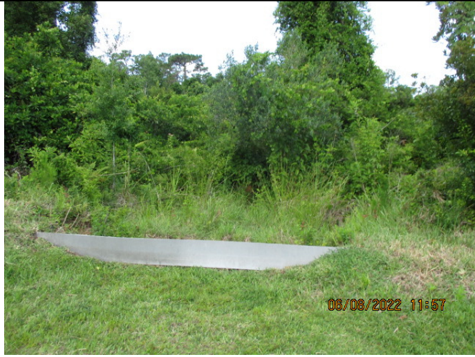
Image 13: Weir, Skimmer road run off, need clearing
