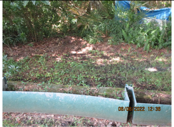
Image 16: Weir Structure, Skimmer west swale, needs clearing
