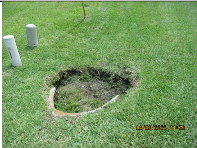
Image 11: FES/Pipe inlet collects water from east boundary flows under road
