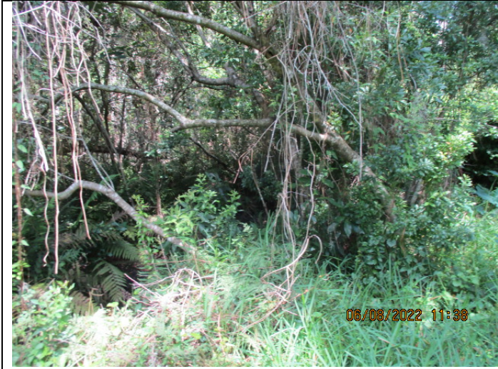
Image 5: Discharge side of weir, needs clearing, possibly re-trenching
