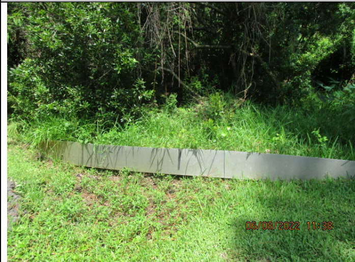
Image 4: Weir Structure & Skimmer at end of swale, discharges to wetland, needs clearing,
