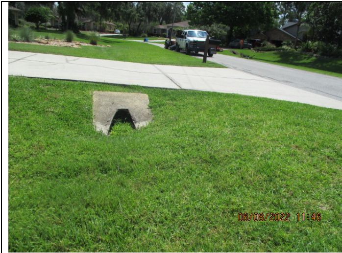
Image 7: MES/Pipe, silt build and vegetation in Roadside swale
