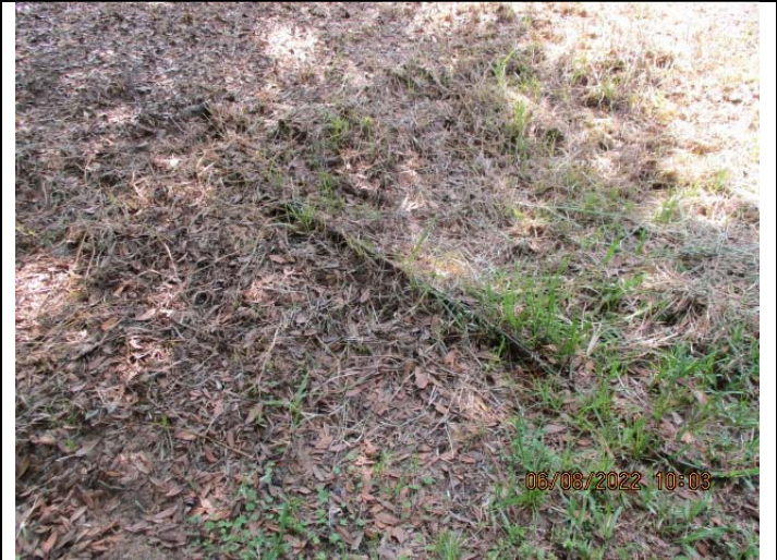
Image 4: Weir, skimmer needs clearing, re-cut swale
