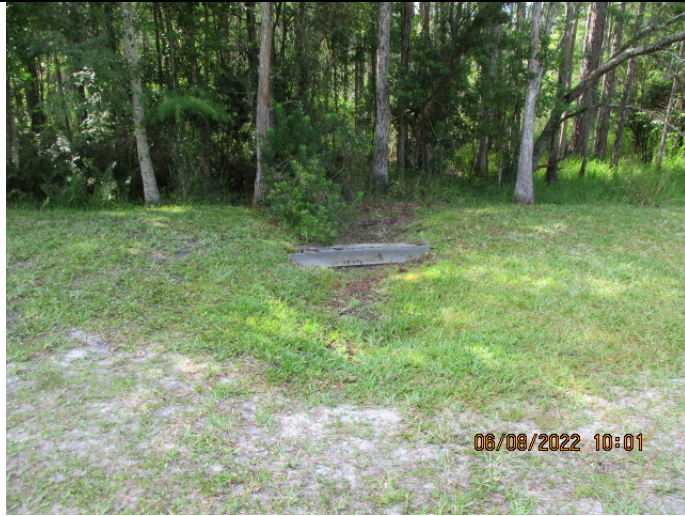
Image 1: : Weir, skimmer needs minor clearing
