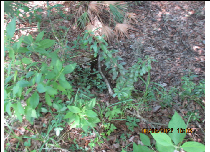
Image 6: Pipe end receives flow from basin, needs clearing, check for obstruction
