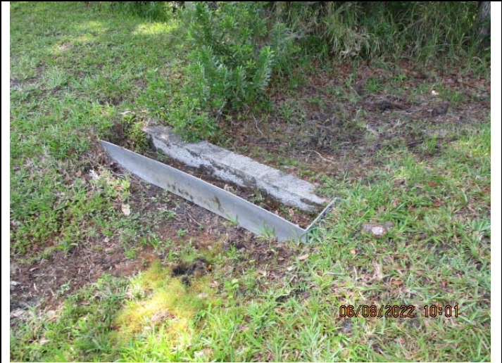
Image 2: : Weir, skimmer needs clearing
